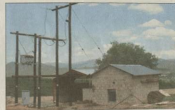
Thanks to funding from the KwaSizabantu Mission, electricity has arrived in the Maqhoko valley.
